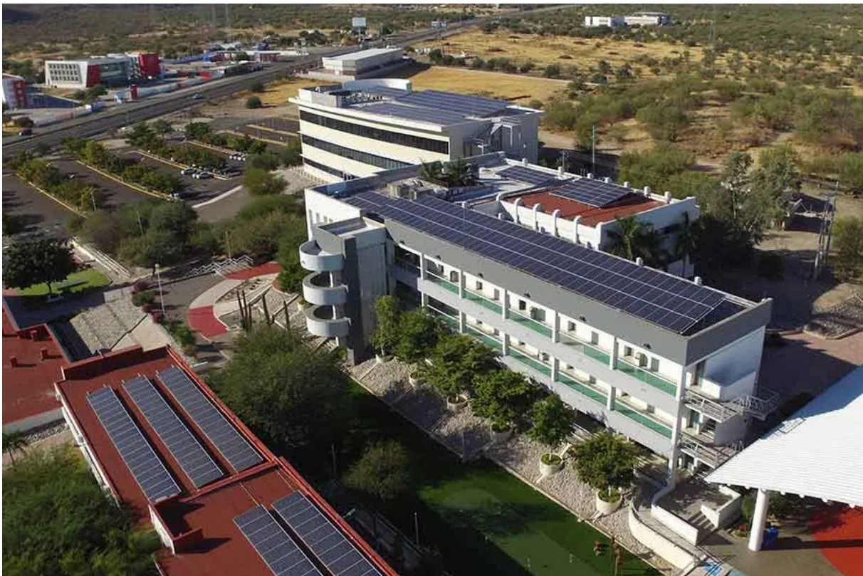
The North Sonora campus' photovoltaic power station.
